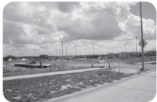
Construction continues on an additional entrance at Elkhorn South High School. Continued on next page
