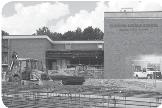
The ramp and landscaping have been removed at Elkhorn Middle School to prepare for the new gymnasium and front entrance remodel.
